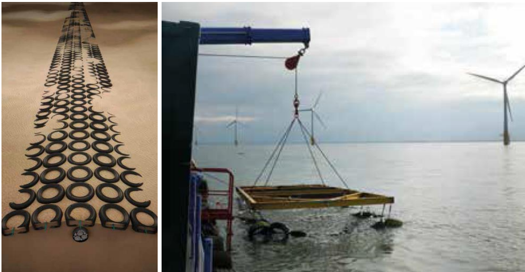
Figure 5.15 (Left) A mattress of rubber tyres used as a cable protection; (right) a mattress being installed with a lifting frame at an offshore wind park ( www.scourprevention.com ).
